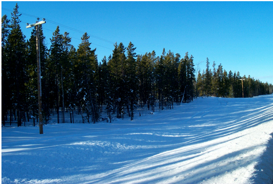
Photo 4-1: Transmission line and right-of-way, Alaska Highway west of Jake's Corner
