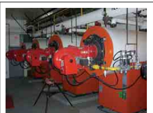
Boilers to heat the hot water for North Vancouver's district heating system are located in a small area of a parking garage. Source: Community Energy Association
