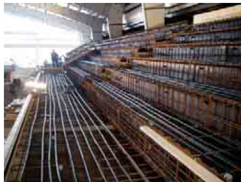
South Cariboo Recreation Centre: Ground-source heating loops to warm the concrete bleachers.
