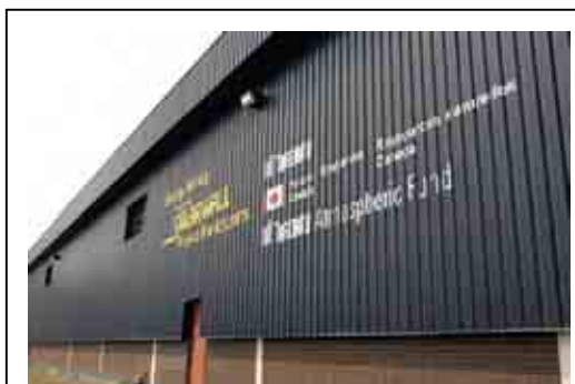
Energy saving Conserval SolarWall on the City of Toronto Vehicle Maintenance Garage. The south wall of the building is covered with 613 square metres of solar cladding. The system has reduced heating costs, enhanced indoor air quality and improved the overall appearance of the building.
