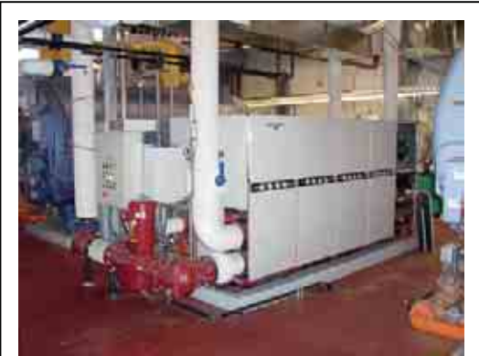
Heat recovery chillers at Okanagan College Source: Community Energy Association
