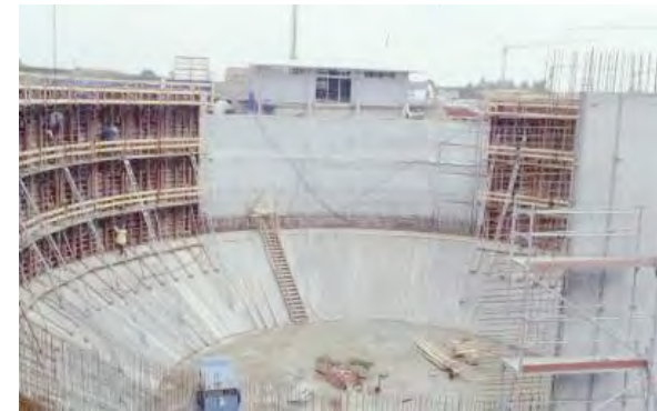
12,000 m 3 seasonal storage, Friedrichshafen, Germany
